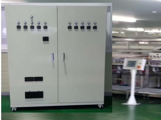
Main Control Panel
