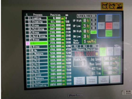
Main Control Screen
