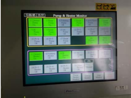
Process Control Screen
